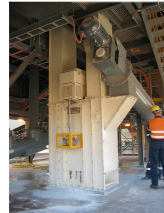
Screw Conveyor feeding a Bucket Elevator
