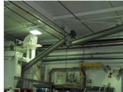
Incline conveyor feeding cross conveyor
